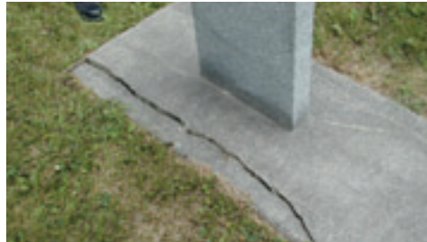
Crack and deterioration of concrete ground beam
